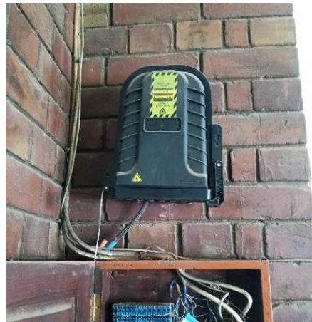
Fibre Optic Box
