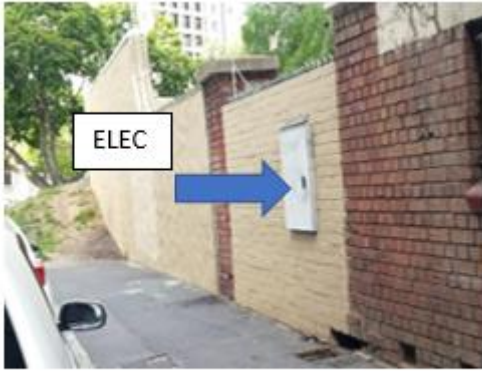
CoCT Electrical supply
