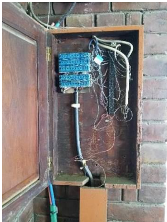
Telkom Distribution Panel
