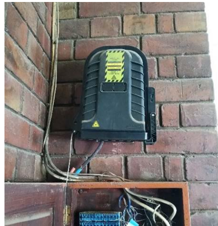
Fibre Optic Box
