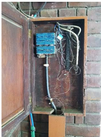
Telkom Distribution Panel
