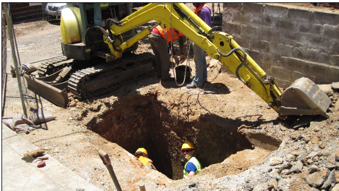
Plate 1: A partially demolished vault was found during the 2014 excavations in trial hole PTL4 (ACO Archive).
