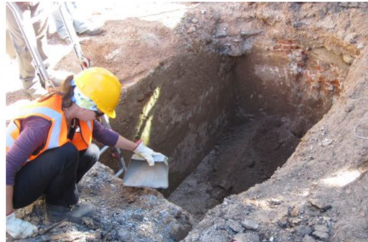
Figure 16 The brick work and lime cement mortar construction of the vault is clearly visible.
