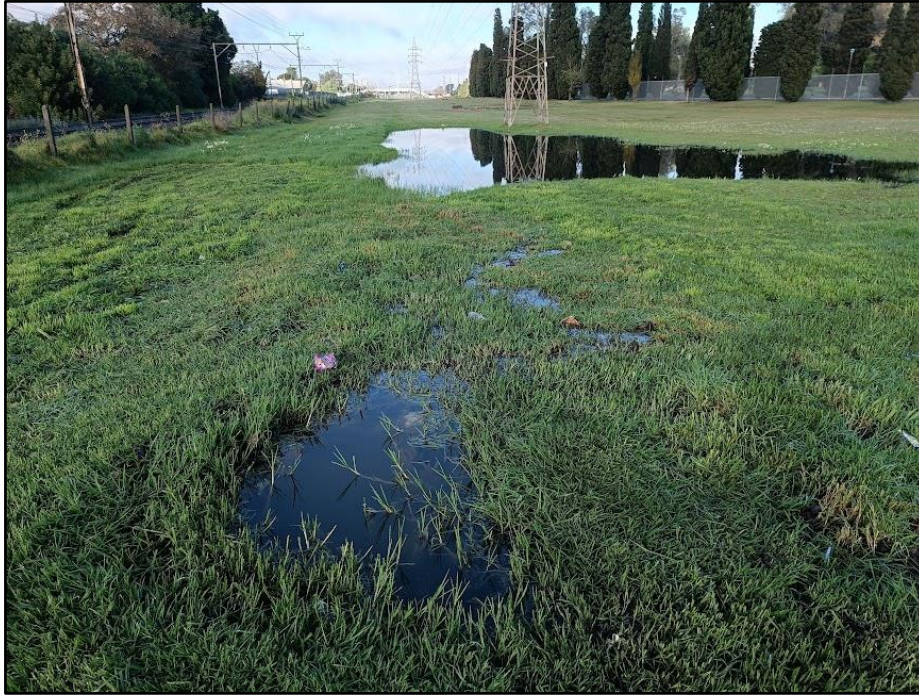
Figure 7.9-11 Ponding visible in the area near the overflowing stormwater manhole.
