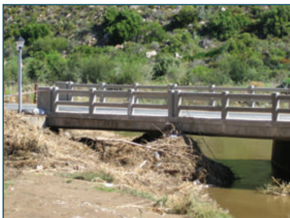
Figure 2.3.2.1: Aggradation beneath the Voortrekker Bridge, Montagu (prior to river works) (Source: Jan Durand)
