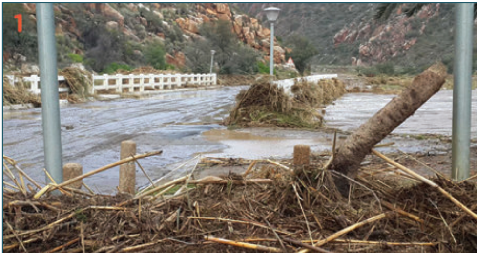
Figure 2.3.2.3: Debris clogging a bridge leading into Montagu (Source: Patrick O’Shea, Adverteyes: http://montagudriedfruitnuts.co.za/montagu-floods-june-2015-keisie-kingna-rivers/ )
