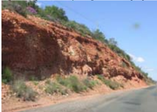
Figure: Slope instability along the Outeniqua pass
