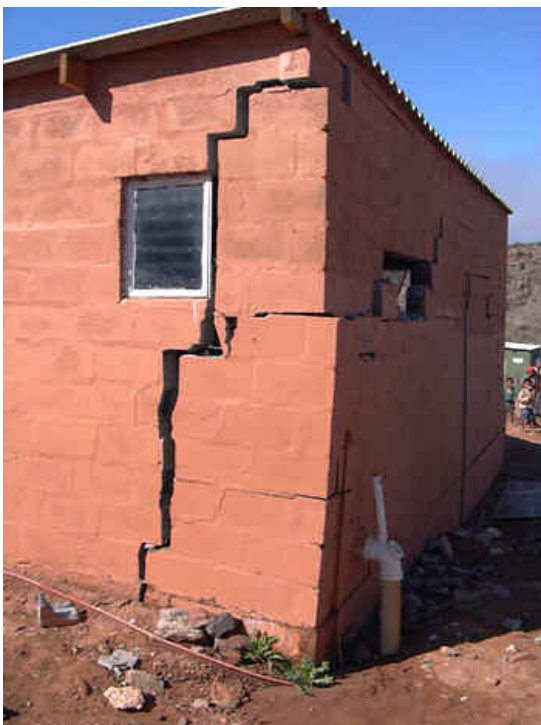
Some of the local houses damaged by the floods, which is part
