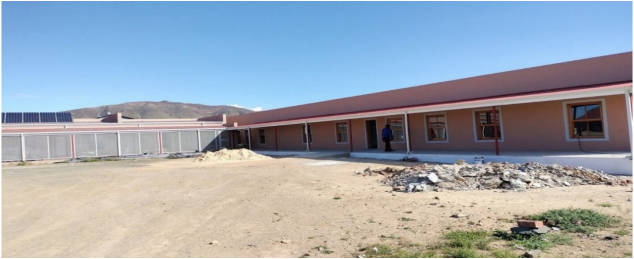
Project Description: Provision of the Prince Albert Municipal Offices at the Thusong Centre
