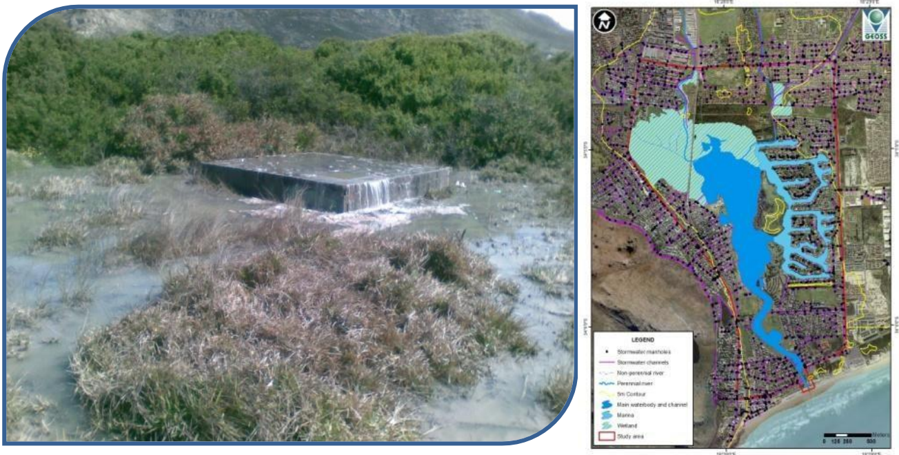
Figure 13: Overflow of sewage pump station in the Westlake area after being vandalized (Sept. 2010) (Courtesy C.Sheasby) (left); and network of stormwater drains around Zandvlei (right)
