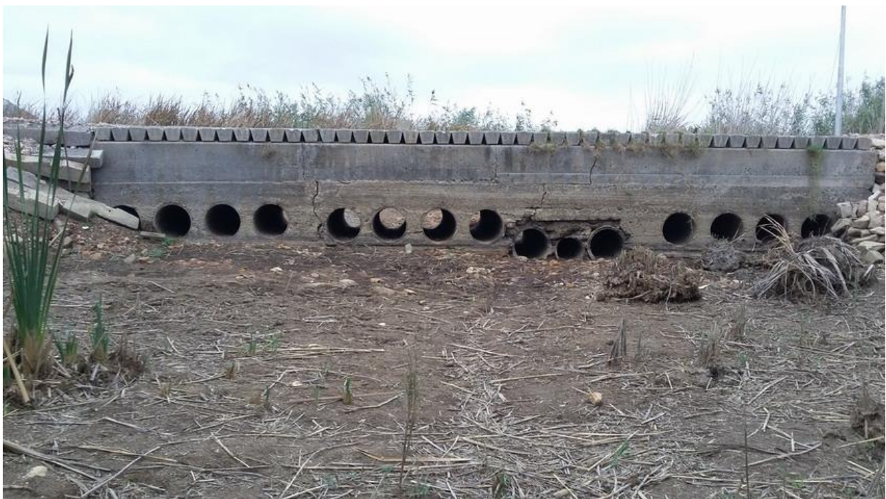
Figure 18: Road crossing creating an obstruction to free-flowing water (Photo: C Malherbe)
