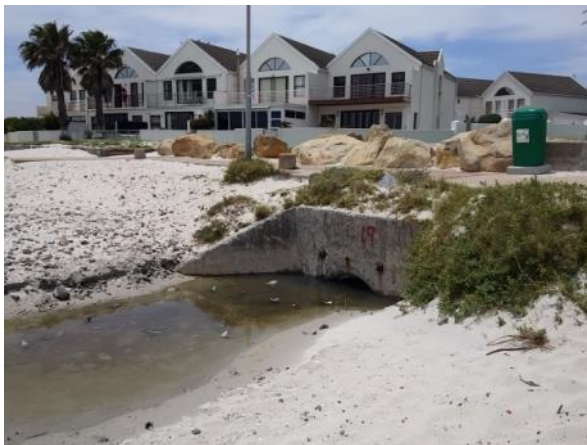
Photo 3: Maintenance of stormwater outlet headwalls and unblocking of outlets is required near the estuary mouth.
