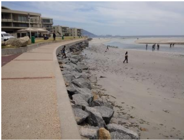
Photo 1: Maintenance of the concrete walkway is required.
