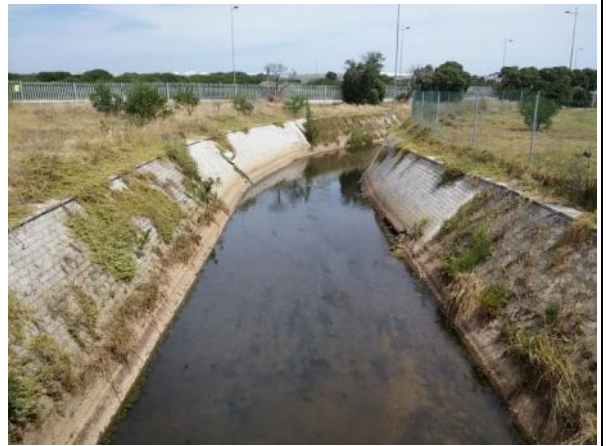
Photo 8: Canals walls at Theo Marais outlet require maintenance.
