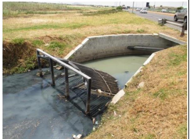
Photo 6: The litter trap at Erica Road stormwater outfall requires maintenance. Note: pollution from sewerage. Removal of litter and other pollution that accumulates at this stormwater outlet and litter trap is also required.
