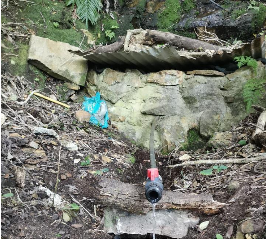
Figure 15: A sump, which collects all the water of a spring, drained by an outflow pipe; the type of structure which can be utilized for the container fill method.
