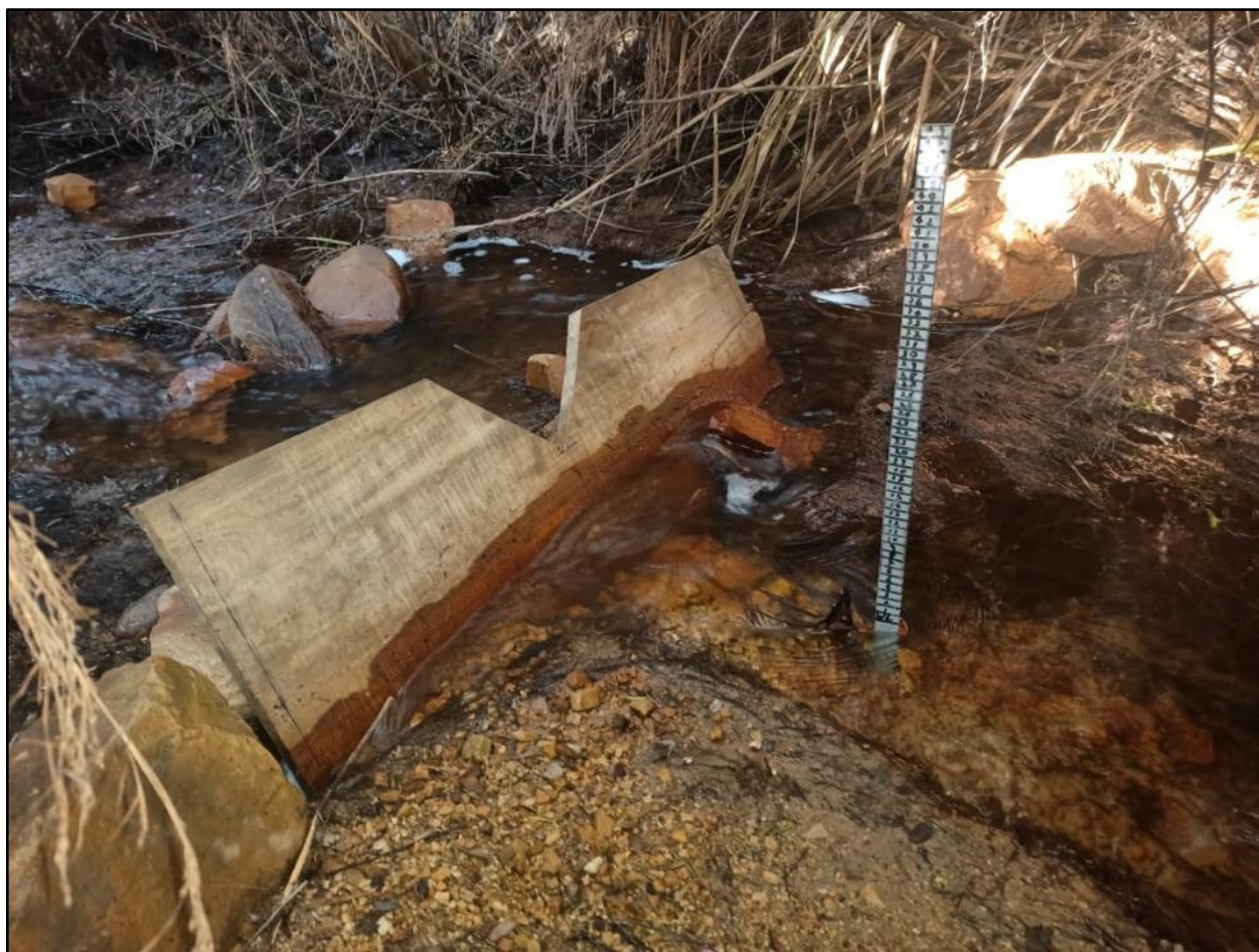
Figure 42: Temporary weir plate compromised after heavy rainfall in the Keurbooms Catchment (Image: Daniel Rogers, 2023).
