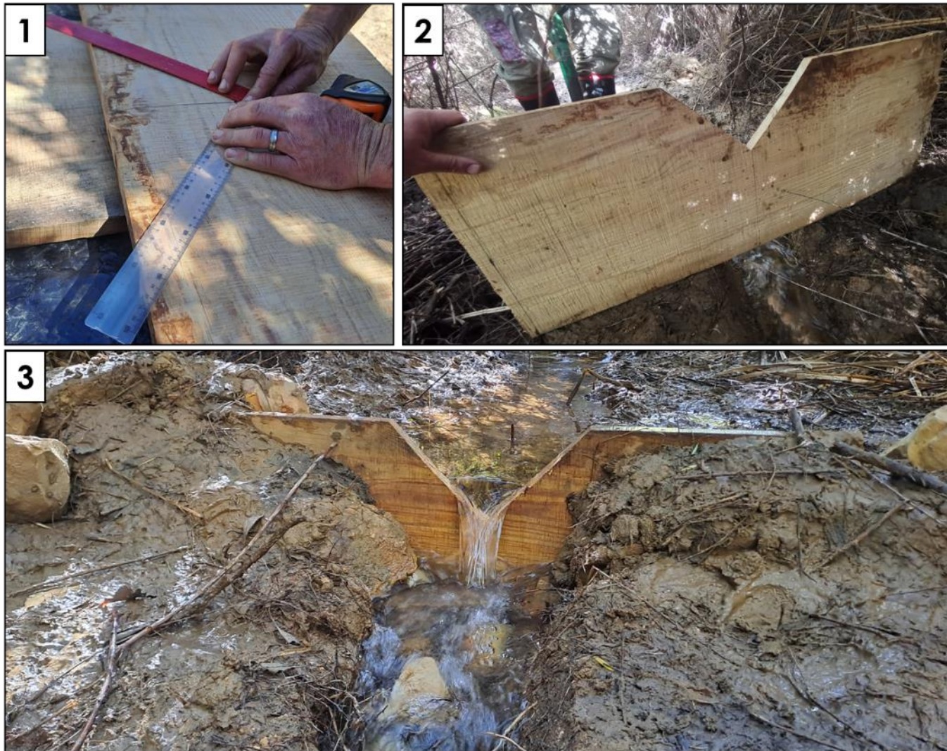
Figure 41: The portable weir method: (1) the weir was constructed in the field; (2) the weir headboard ready for implementations; (3) and the weir being tested in the field.
