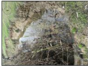
SCOUR DAMAGE DOWNSTREAM
