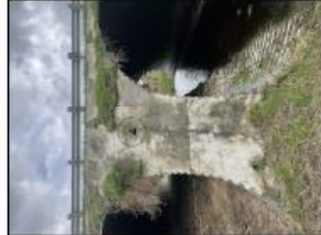
CRACKS IN CONCRETE
