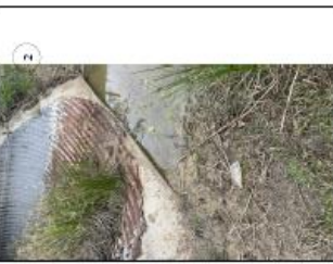
SCOUR DAMAGE UPSTREAM
