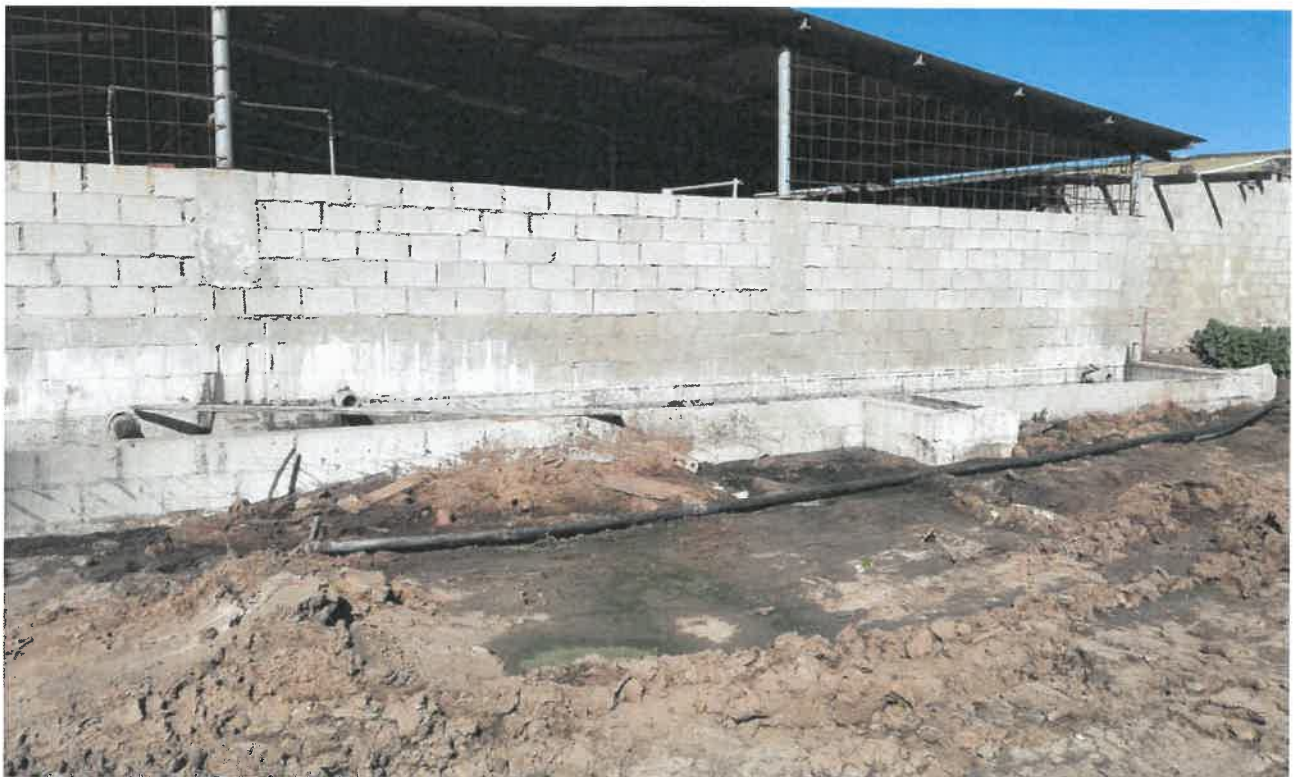
Photo 2: The cement holding tank located behind the new shed showing seepage into the soil.
