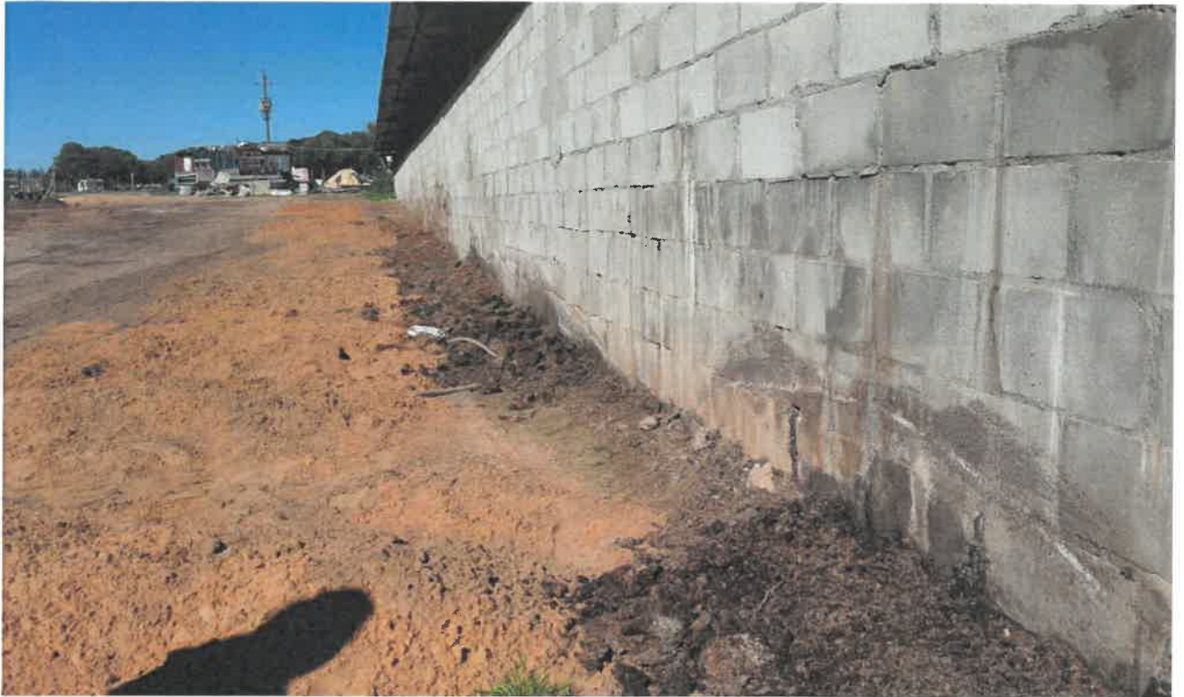
Photo 1: Effluent and sludge seeping through the walls of the new shed.
