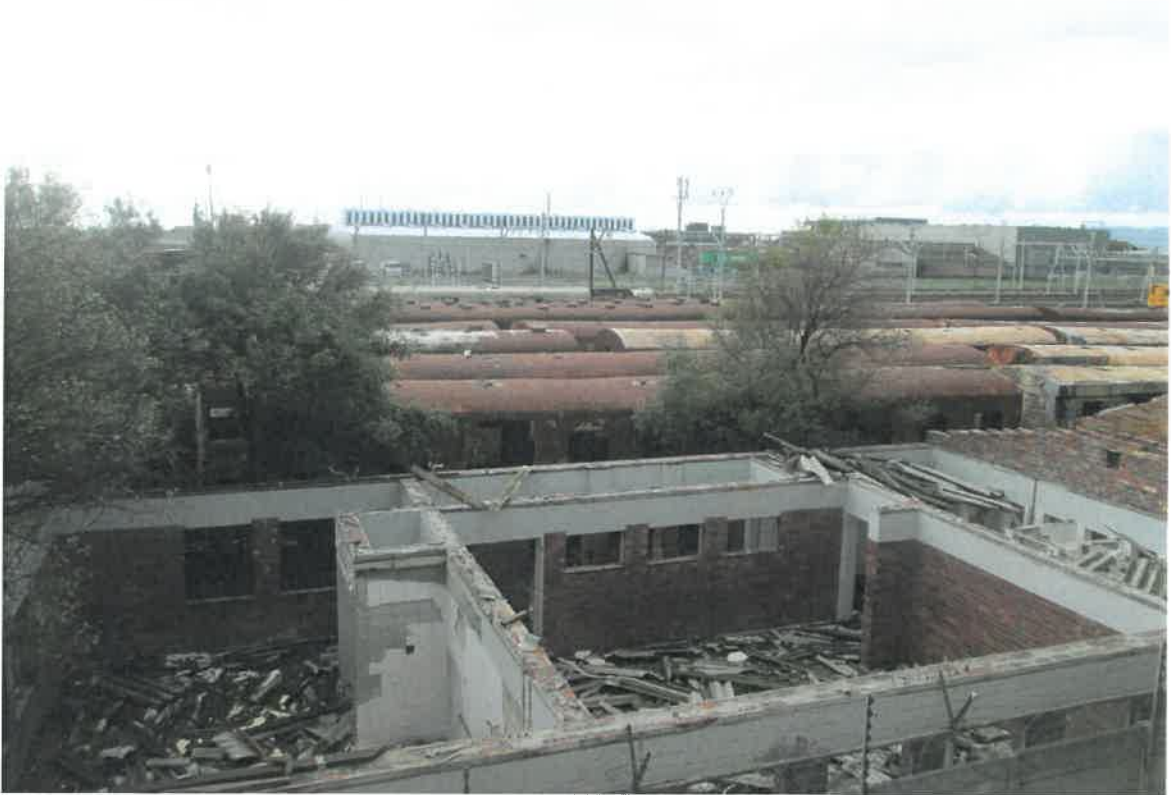
Photo 1: View of the collapsed asbestos roof of PRASA's old building.
