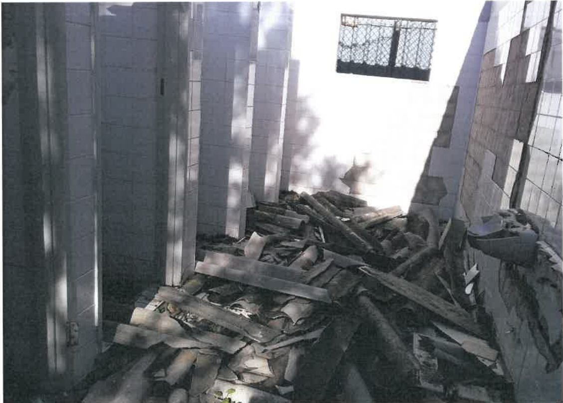
Photo 4: Asbestos left unattended
