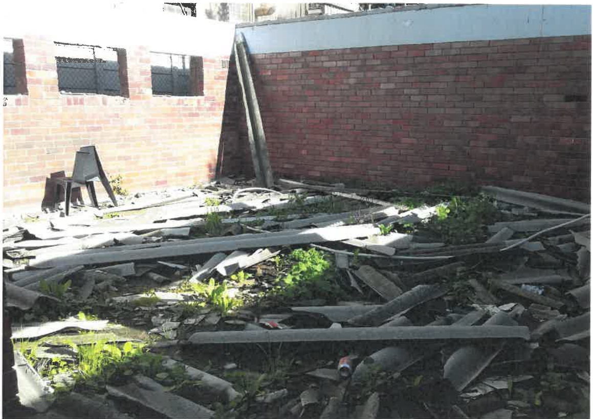
Photo 2: Asbestos left unattended.
