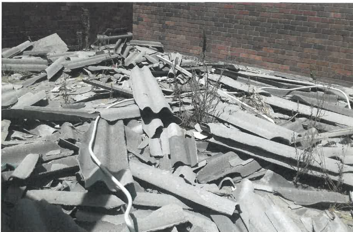
Photo 5: closer view of asbestos left unattended.
