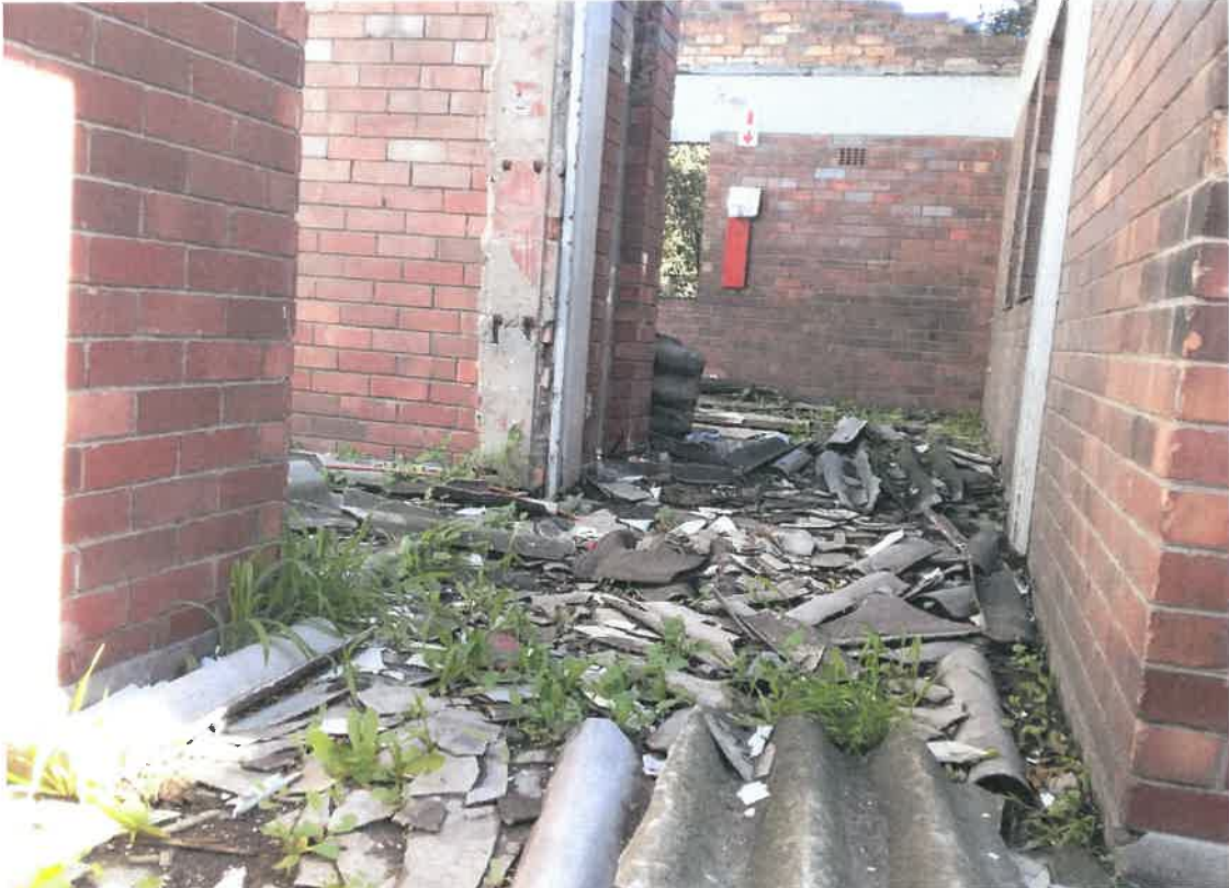
Photo 3: Asbestos left unattended
