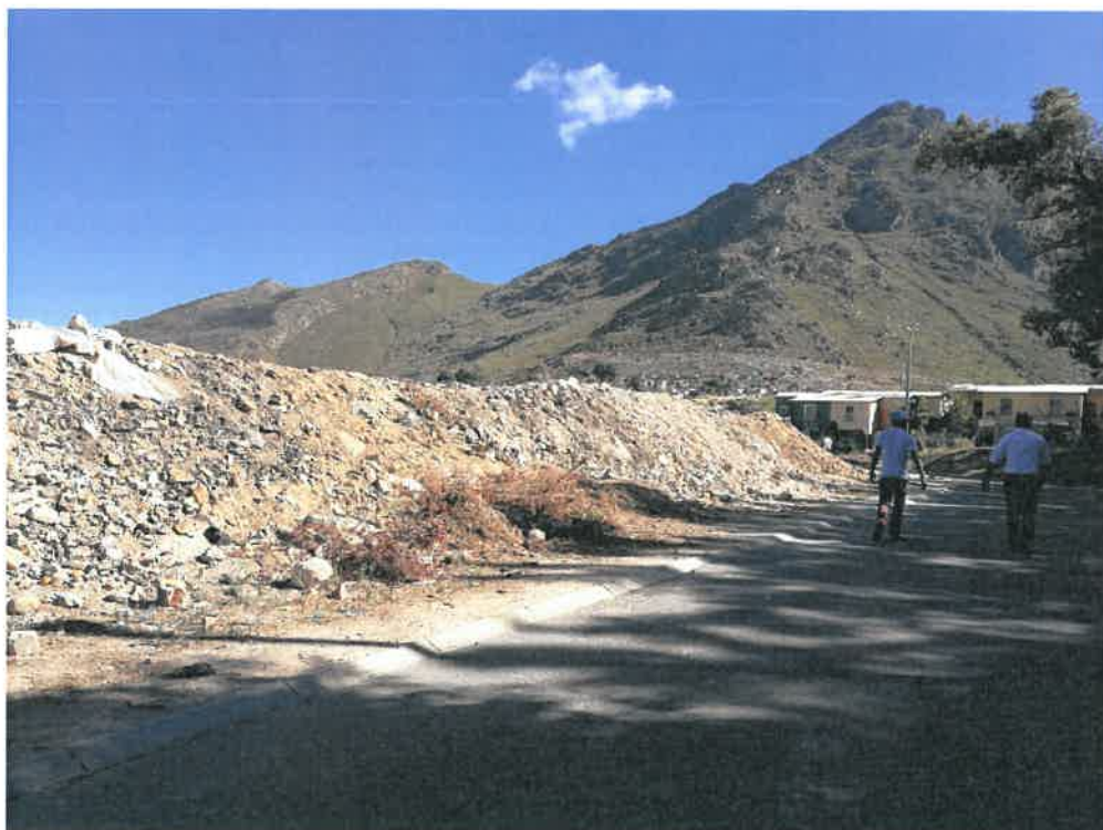
Photo 3: Disposal of inert waste to develop a sand berm which is adjacent to Le Roux Road.
