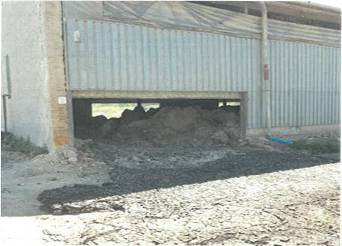
Photo 4: Seepage of wet chicken manure from beneath chicken house.
