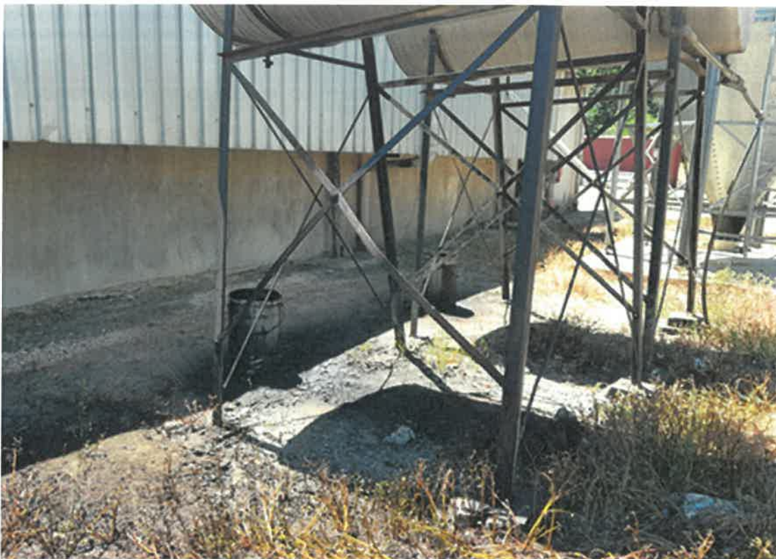
Photo 8: Unbounded fuel/oil storage tanks and spill of oil on the ground on the property.
