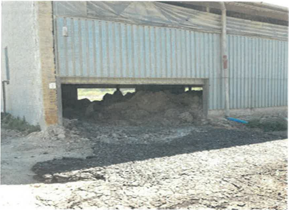
Photo 4: Seepage of wet chicken manure from beneath chicken house.
