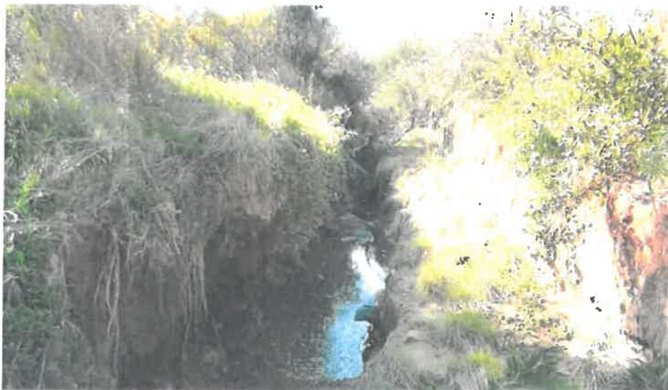
Photo 3: View of the channel that was constructed to divert the water away the Efflux Cave opening, now eroded wider and deeper.
