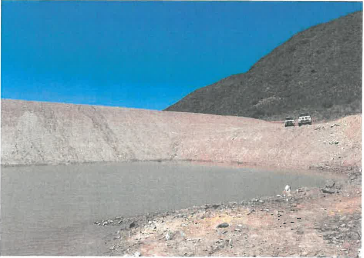
Photo 2: Alternative view from the expanded dam.
