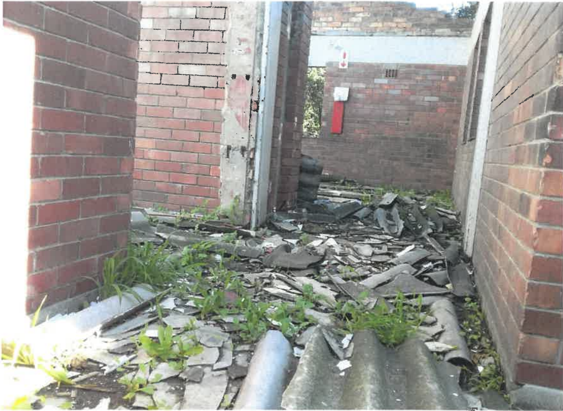
Photo 3: Asbestos left unattended
