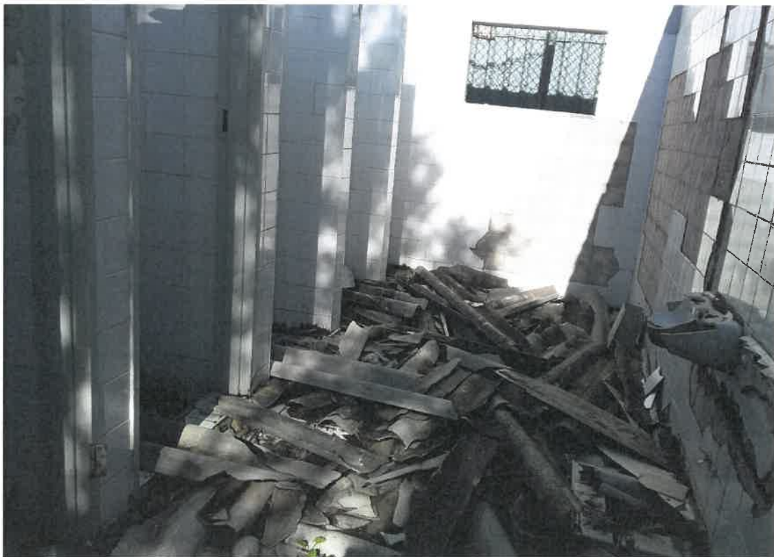
Photo 4: Asbestos left unattended
