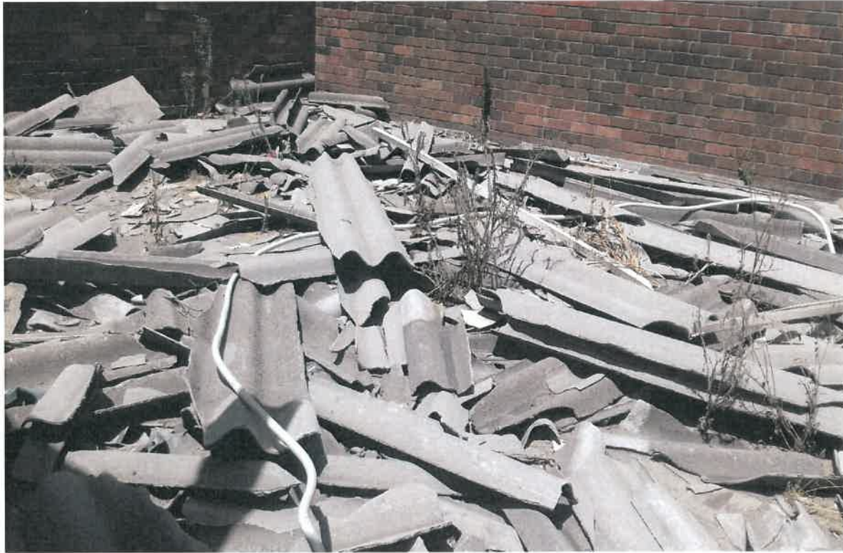
Photo 5: closer view of asbestos left unattended.
