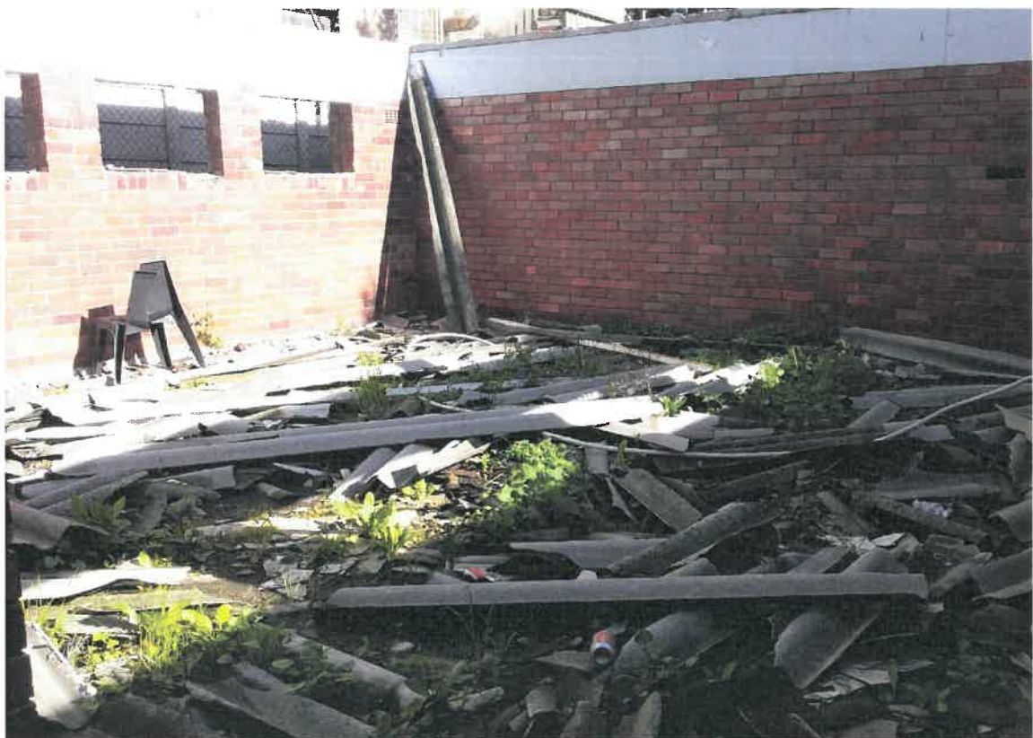
Photo 2: Asbestos left unattended.
