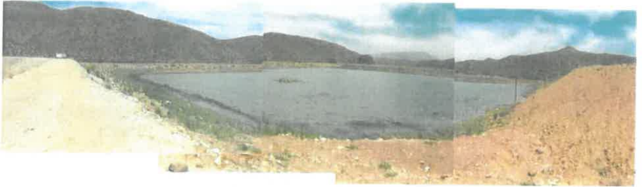
Photo 4: Expansion of a dam on Farm Buffelskloof 16/97, Ladismith. Combined capacity of all the dams expanded believed to be more than 50 000 cubic metres.
