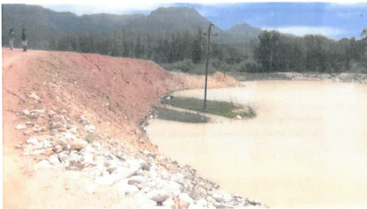
Photo 5: Height of dam wall increased by 2.5 metres or more on Farm Buffelskloof 14/97, Ladismith.
