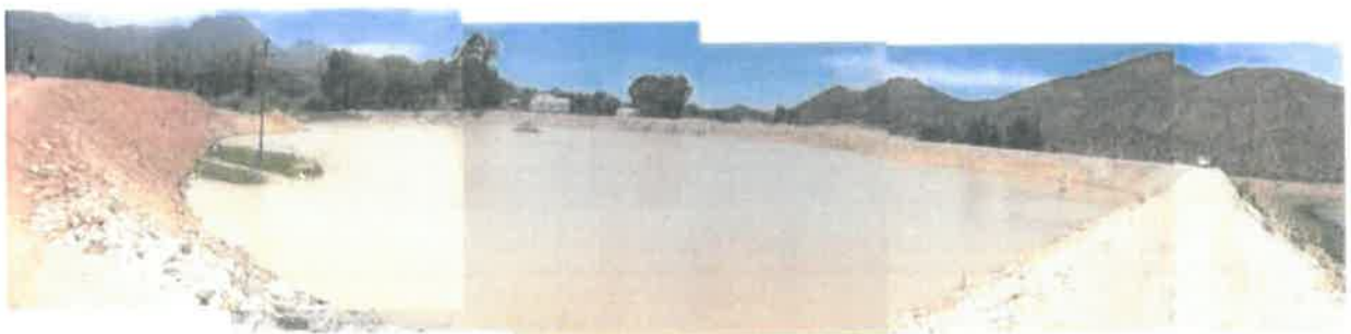
Photo 3: Expansion of a dam on Farm Buffelskloof 14/97, Ladismith. Combined capacity of all the dams expanded believed to be more than 50 000 cubic metres.
