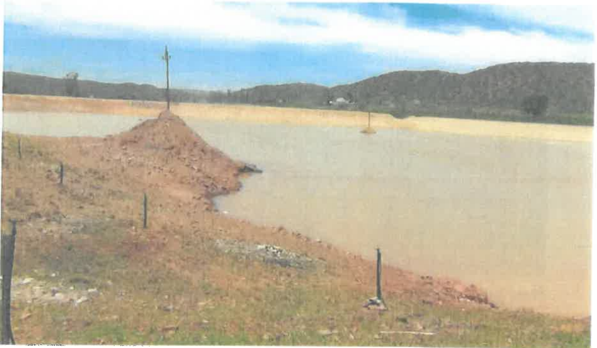
Photo 1: Development and or expansion of a dam on Farm Krantzkop 4/100, Ladismith exceeding 100 square metres within 32 metres of a watercourse (Dwars River).
