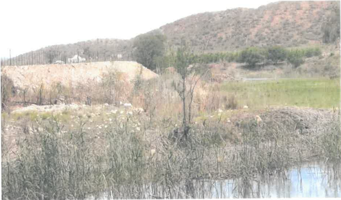
Photo 2: Development of a dam on Farm Krantzkop 4/100, Ladismith exceeding 100 square metres within 32 metres of a watercourse (Dwars River).
