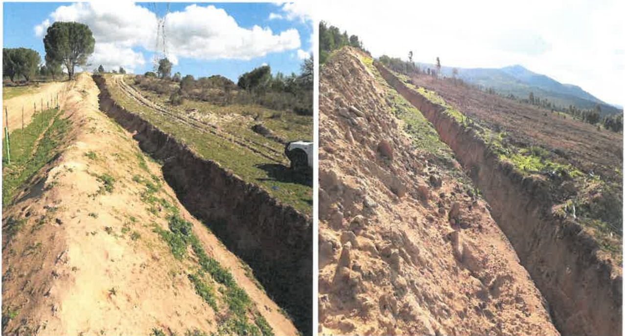
Photo 1-2: Clearing of more than 300m 2 of indigenous vegetation and the development of canals exceeding 10 square metres in size
