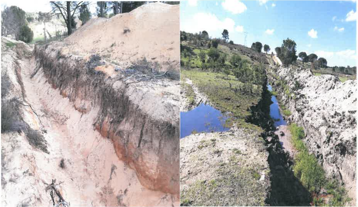
Photo 3-4: Moving of soil and sand of more than 5 cubic metres in size from a watercourse
