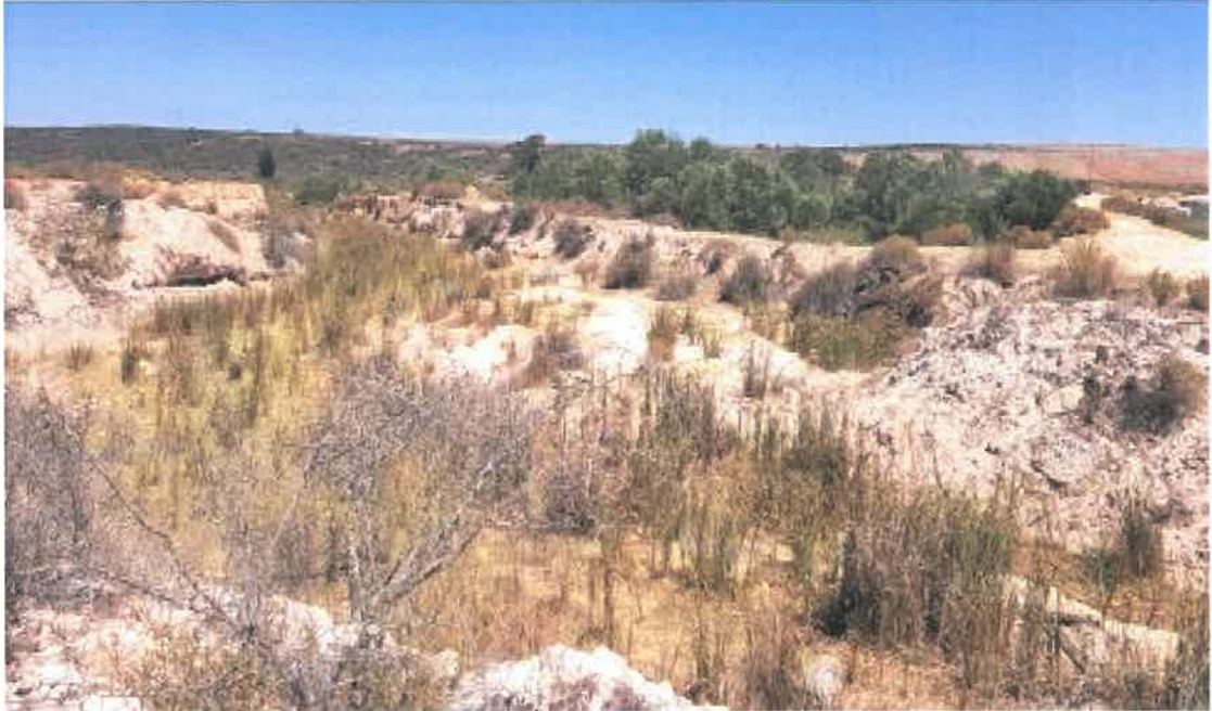
Photograph 3: Area where erosion adjacent to the dam wall had occurred.
