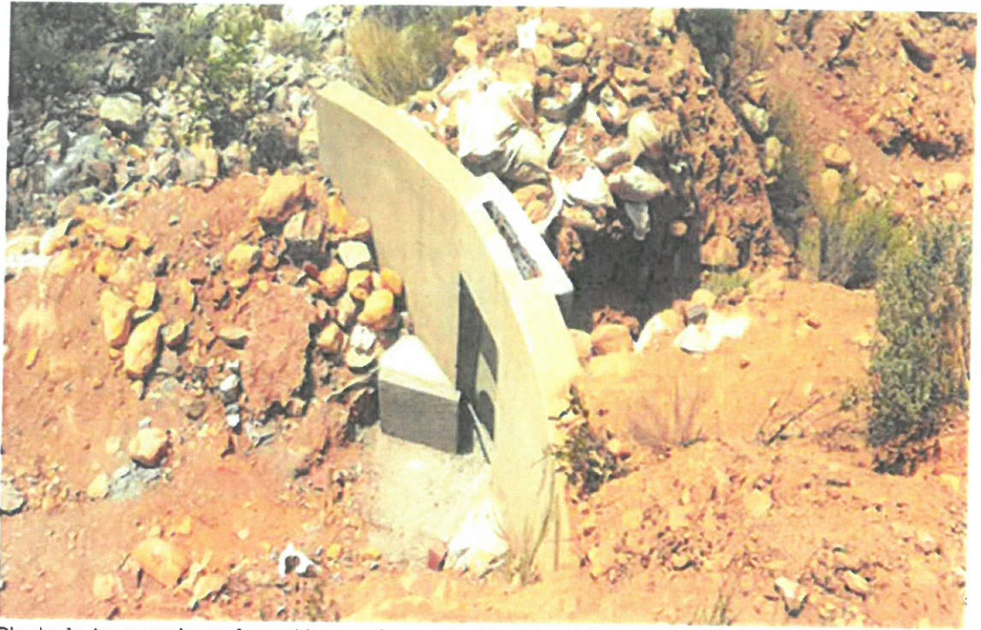
Photo 1: An overview of sand bags placed behind the sluice and material and rock laced in front of the sluice within the river bed.
