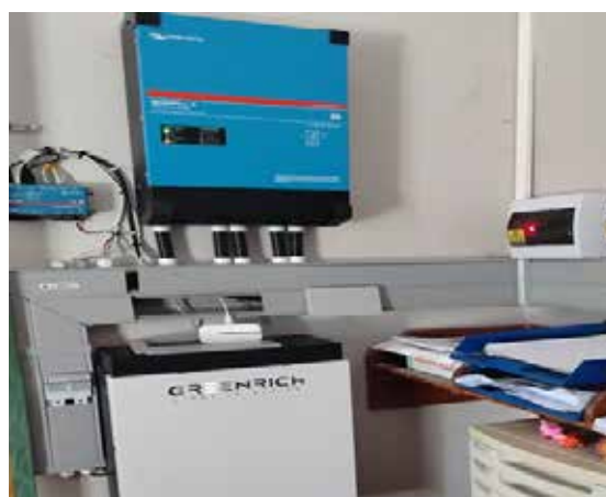
Inverter system to the CCTV system at GD facility.
