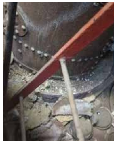
Figure 3: Damaged heat pump.
