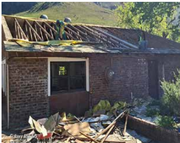
Breach of safety regulations: workers on the roof without harnesses, compromising safety.
