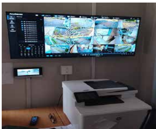
Monitoring via the CCTV camera system at GD facility.
