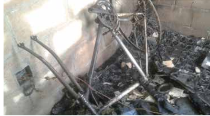
A number of the households’ belongings were damaged or destroyed.
