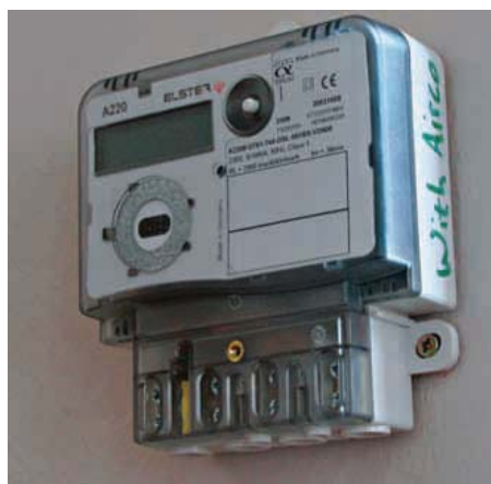
AN INTELLIGENT ENERGY LOGGER INSTALLED AT THE DEPARTMENT BUILDING.
