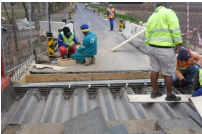
Work on rehabilitating a steel bridge over the Breede River near Bonnievale.
