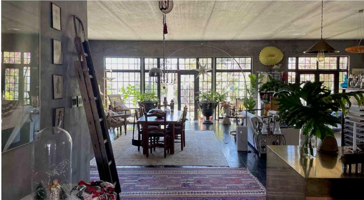
The largely gutted interior with new precast plank ceiling/first floor and new doors & fenestration on the Alexander Road side of the property.
