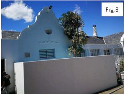
Note that the window of the nearest gable has been replaced and is completely different to the remaining original window in the other gable. (Noted as 'Work not done' in Heritage Report, p.14).
