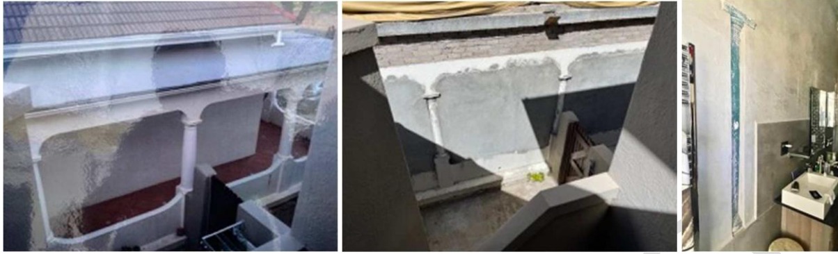
Left: The side stoep prior to enclosure (center). Far right: Part of this enclosure now accommodated an ensuite bathroom in which surviving embedded columns are still partially visible.
