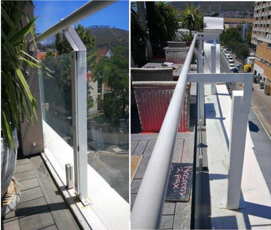
Fig.6 and Fig.7 show the relationships between parapet, frameless glass and steel structure.
