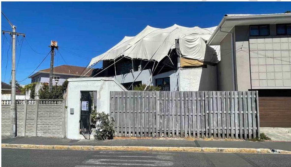
View of the building from Alexander Road. Note proximity of the corner of the neighbour's projecting eaves.
