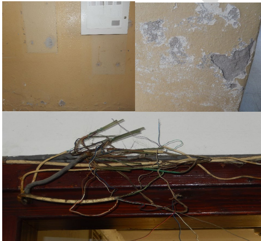
FIGURE 5: Damp in the walls and bad electrical wiring
