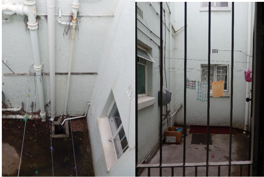
FIGURE 4: Small inner courtyards with an aging plumbing system, use for laundry
