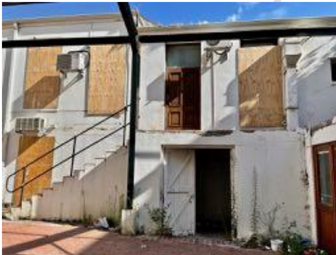
FIGURE 03: Boarded up fenestration at the back of the former NICRO building. Note the good surviving teak four panel door with fanlight.
