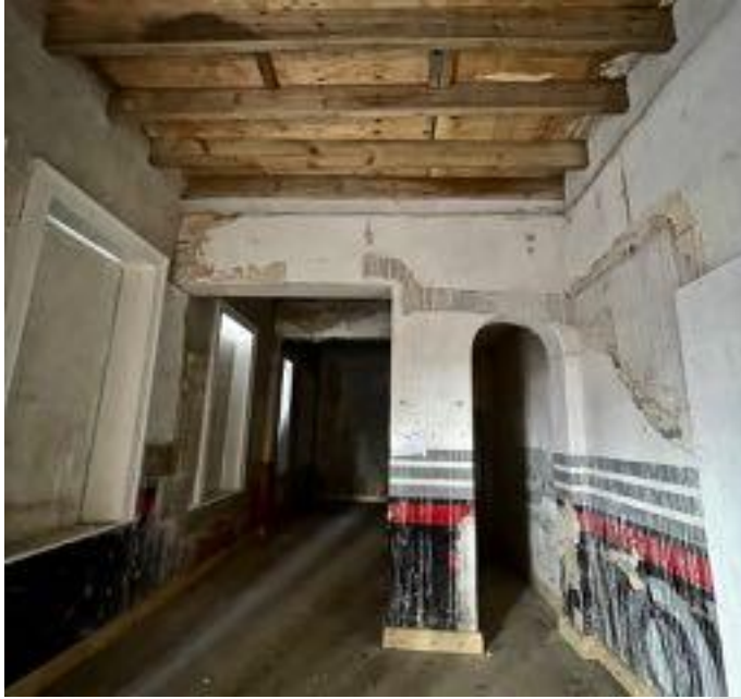
FIGURE 02: The corner building interior on the ground floor. This was the only interior on the property that was accessible.
