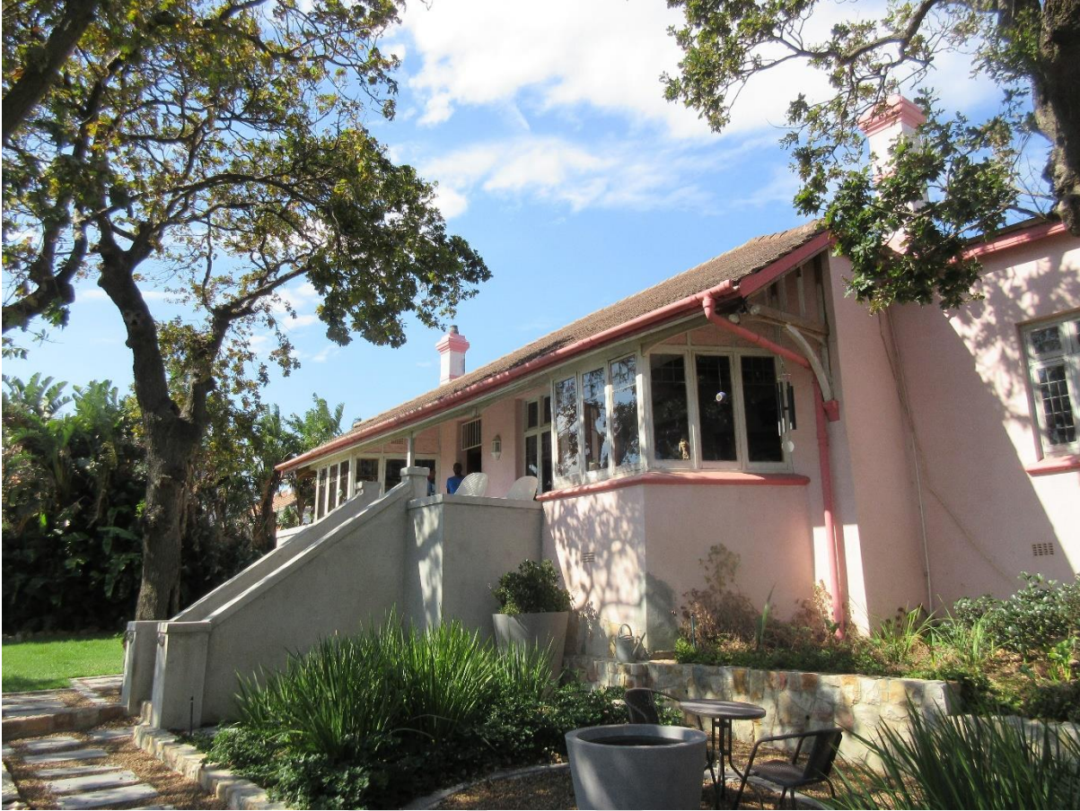
The elevated veranda protected by its position between the two bay windows, which to improve functionality has seen one post sacrificed.
