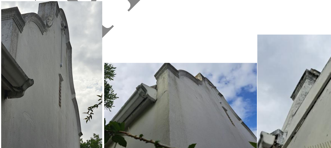
Figure 10 (below right): Detail view of chimney facing neighbouring property (10 Rochester) that has been blocked up and not in use.
