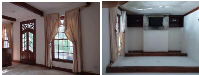
Front NW bedroom – fireplace Interior view of NE facing door & windows Main reception room with fireplace, proposed wall removal
