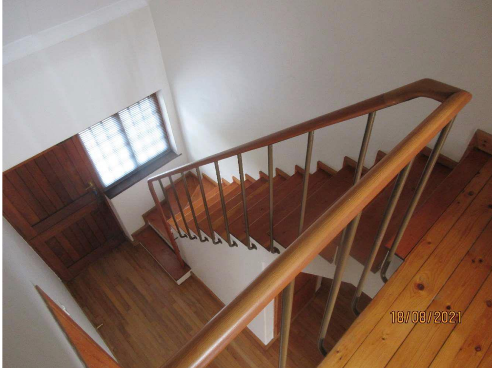
View of vestibule and staircase from the landing/bridge of the 1st floor. Note the delicate mop-stick handrail of Oregon Pine, natural and unpainted, on steel balusters fixed to the side of the outer (well) string, which coincident with the turn/ change in direction affected by winders, transforms to become a newel.
