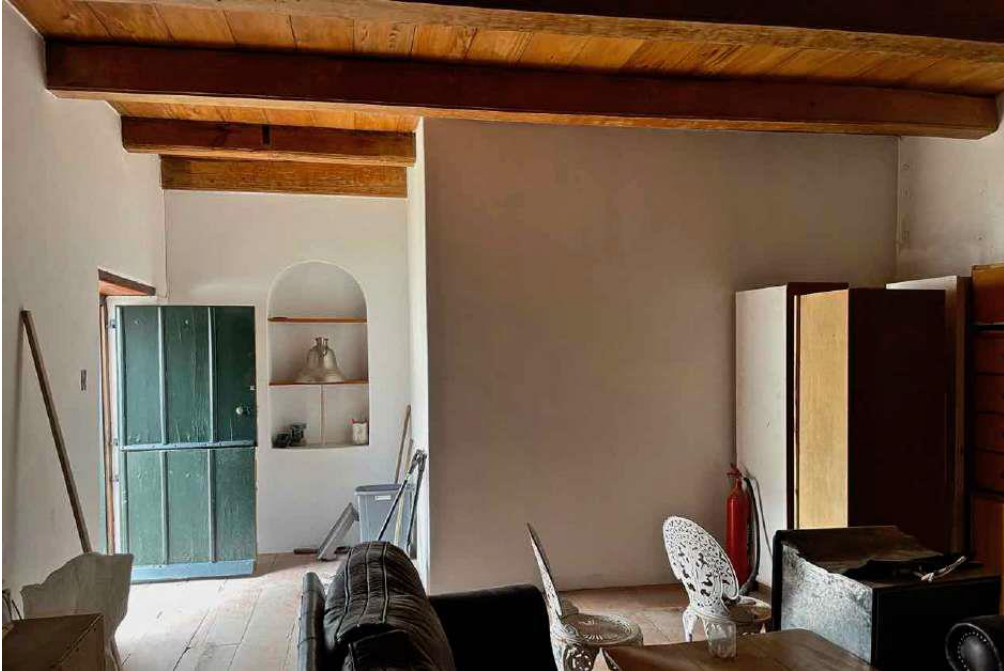
En suite bathroom insertion into central sitting room around ceiling rafters and up to ceiling boards. Removed Fagan kitchen cupboards stored on the right.
