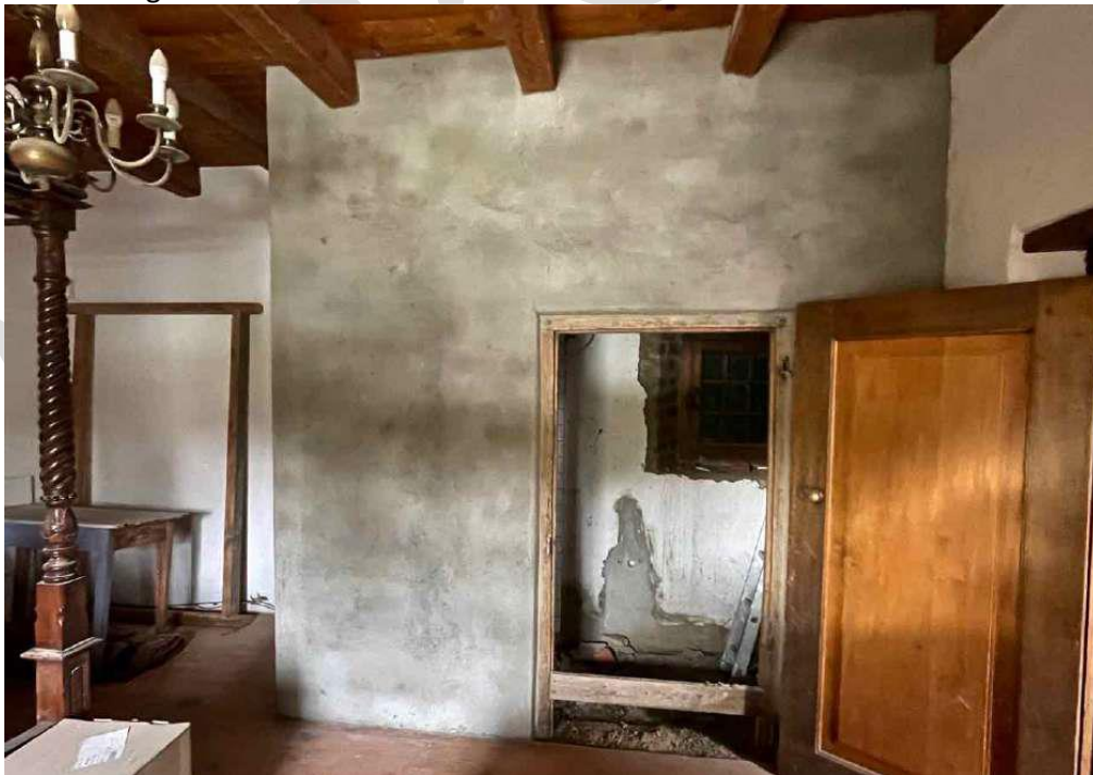
En suite bathroom insertion into front bedroom around ceiling rafters and up to ceiling boards.
