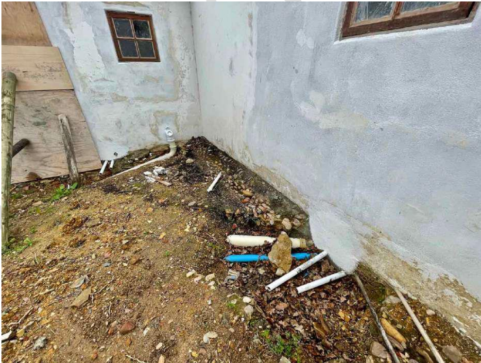
Back yard: Fagan era cobbled yard and drainage channels to be displaced without detailed proposals of their replacements.
