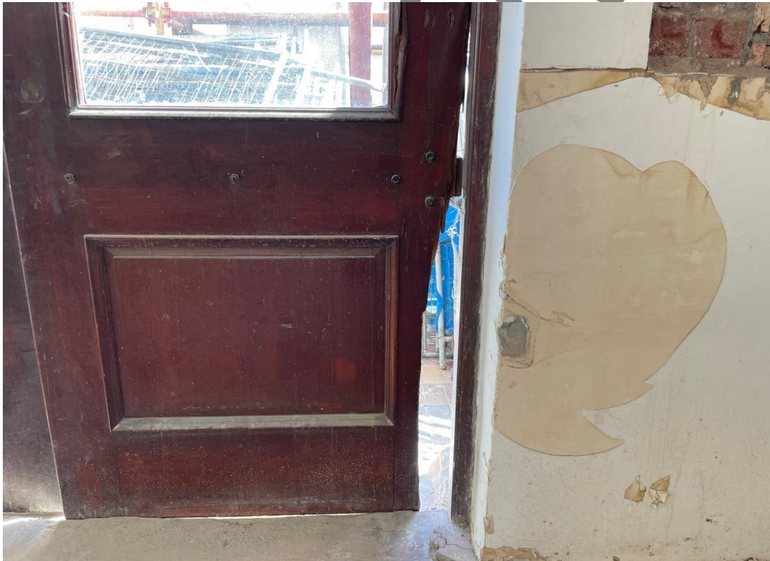
Figure 2 – A Damaged door in the Union Castle Building
