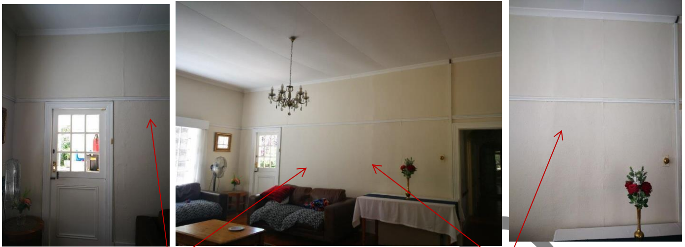
Figure 8: Living Room : Evidence of original / earlier walls that have been demolished (indicated by red arrows) can clearly be seen. These walls may have been removed at the same, or different, times to create the current larger space forming the western forward projecting gabled room. The cottage pane glazed door in the corner leads to the existing covered veranda.
