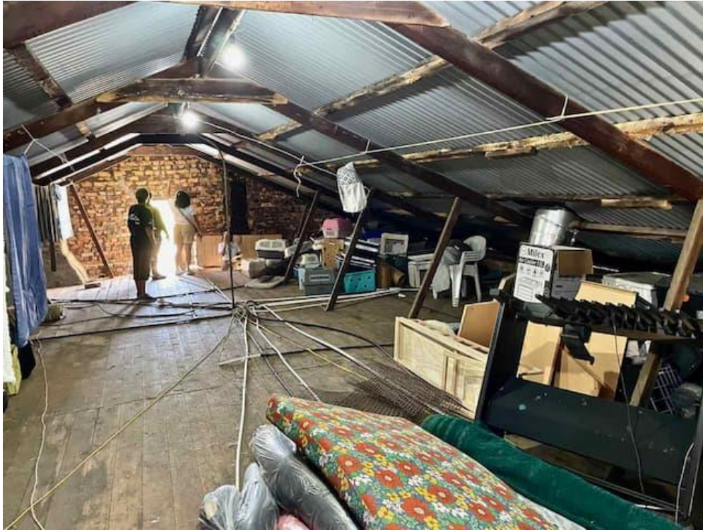
FIGURE 04: Loft space with typical latter 19th/early 20th C era collar & twinned web trusses (no kingposts). The loft floor is part of the ceiling viewed from ground level.
