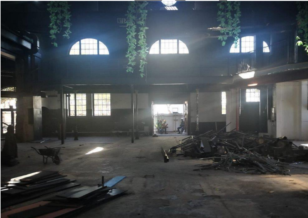
Figure 4 – Interior of the Power Station Building showing the clearing out of previous installations in progress.
