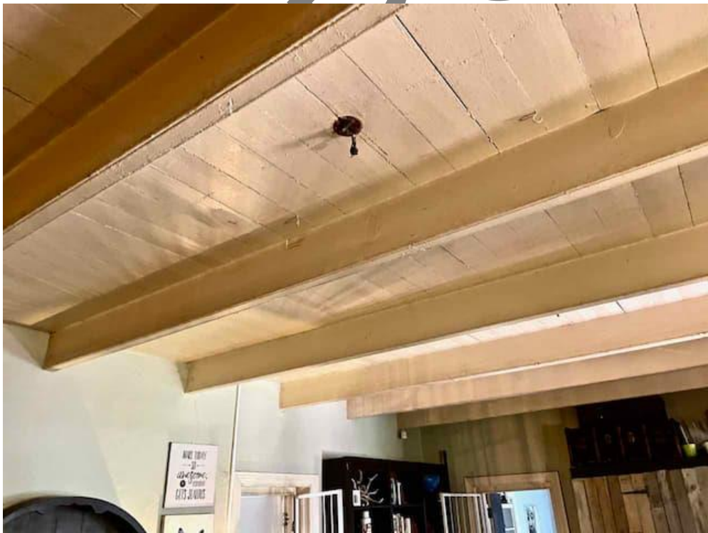
FIGURE 05: Timber board ceiling supported on latter 19th/early 20th C quirk & bead profiled rafters.
