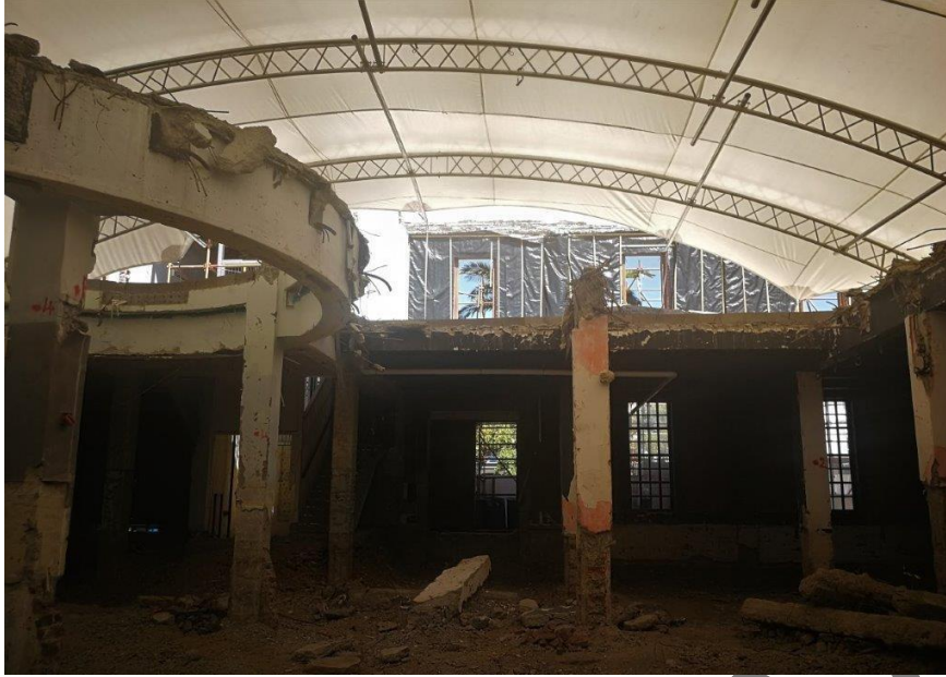
Figure 1 – Interior of the Union Castle Building with the protective temporary roof and plastic sheeting applied to the interior surface of the walls.
